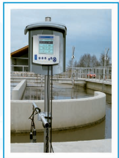
Continuous online effluent monitoring system
